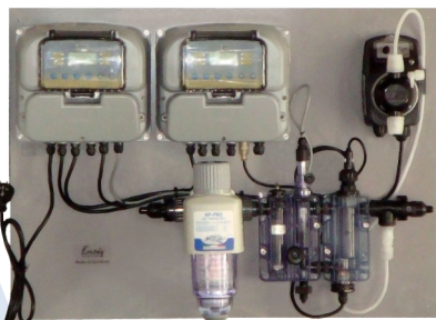
Chlorine Dosing and pH with Self Cleaning Pre-Filter
