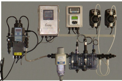
Chlorine Dioxide Dosing, pH Neutralisation Turbidity Monitoring with Recording and Data Logging
