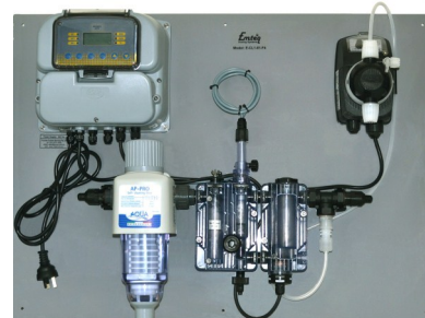
Chlorine Dosing with Self Cleaning Pre-Filter
