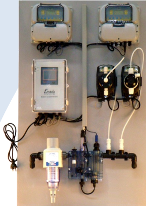
Chlorine Dosing and pH Correction with Data Logging
